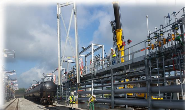
Rail Loading Facility
